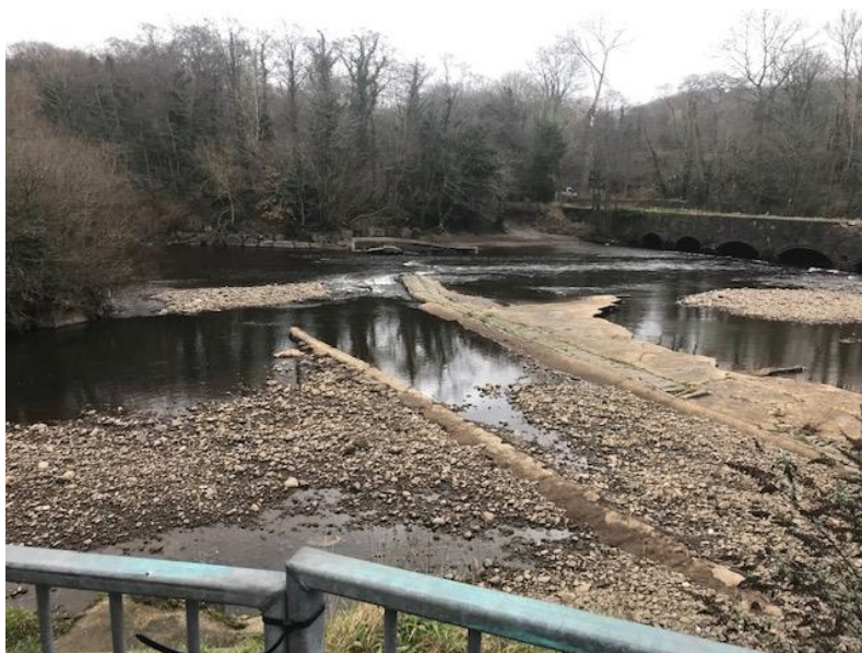
Figure 2 - View of remaining weir and inlet channel showing sediment build up.
