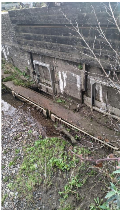
Figure 3 - Penstocks at inlet to channel feeding the Tennant Canal – clearly non-functional due to stone/sediment accumulation.
