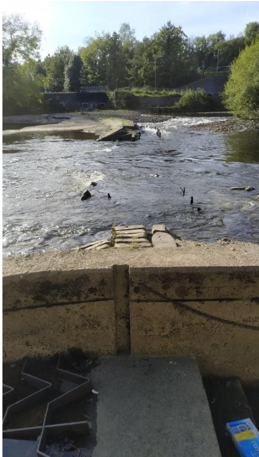
Figure 5 - View along the damaged weir from the fish pass on the Eastern bank showing breach of the weir.
